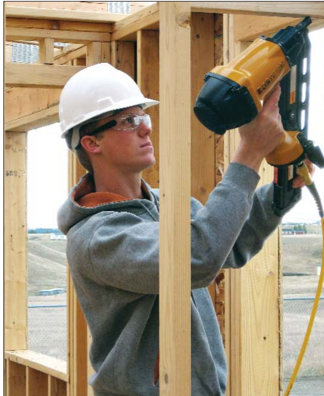
In order to learn professional construction skills, D.J. Kamp and two dozen other high school students are building a 3-bedroom modular home.
