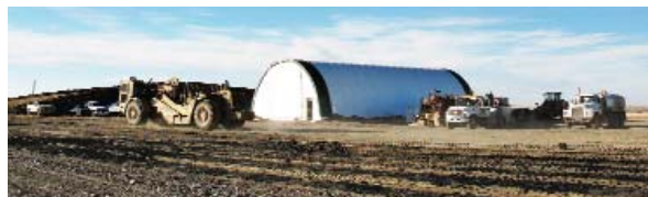
Wickens Construction of Lewistown started site preparation in October. Photos by Tim Gregori and Marvin DeBuff.
